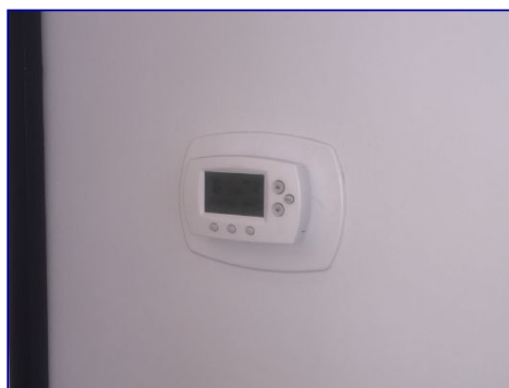
The furnace thermostat is on the dining room wall.
