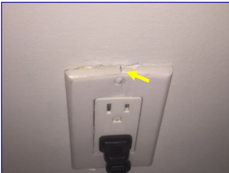
There was al broken cover plate for the electrical receptacles in the front bedrooms of the home.
