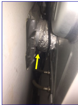
Laundry dryer vent.
