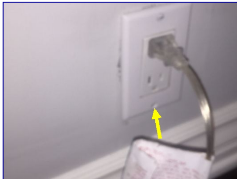
The electrical receptacle in the dining room back wall is missing a screw.
