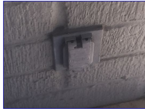
The left side electrical receptacle on the back patio was not GFCI protected.
