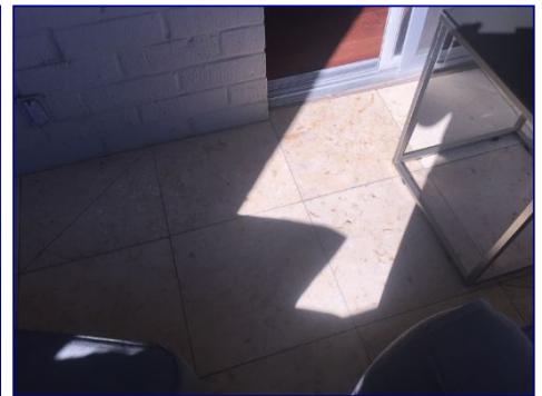
The back patio tiled flooring is not slip resistant. May have issues when wet.
