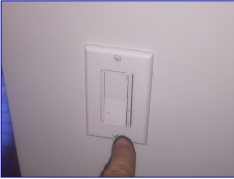
Dining room dimmer switch did not dim the light.
