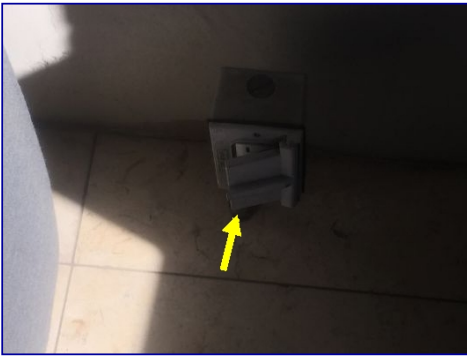
The back patio GFCI receptacle had no power and needs a new cover.
