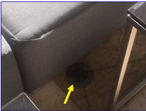
Floor drain drains to the exterior wall.
